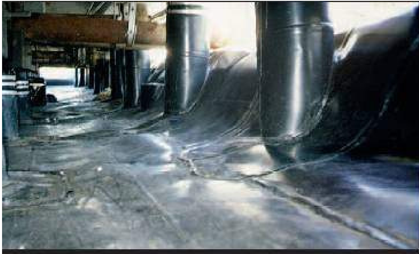
Secondary containment for ground water protection
